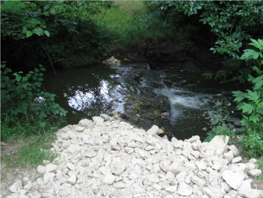
Standing on the west bank, looking east, after Sewer Maintenance made a temporary repair to stabilize the pipe.
