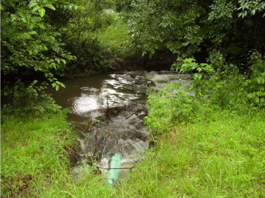
Standing on the west bank, looking east. Approx. 10 lf of pipe was exposed to the west of the existing encasement and cut-off wall. (June, 2007)
