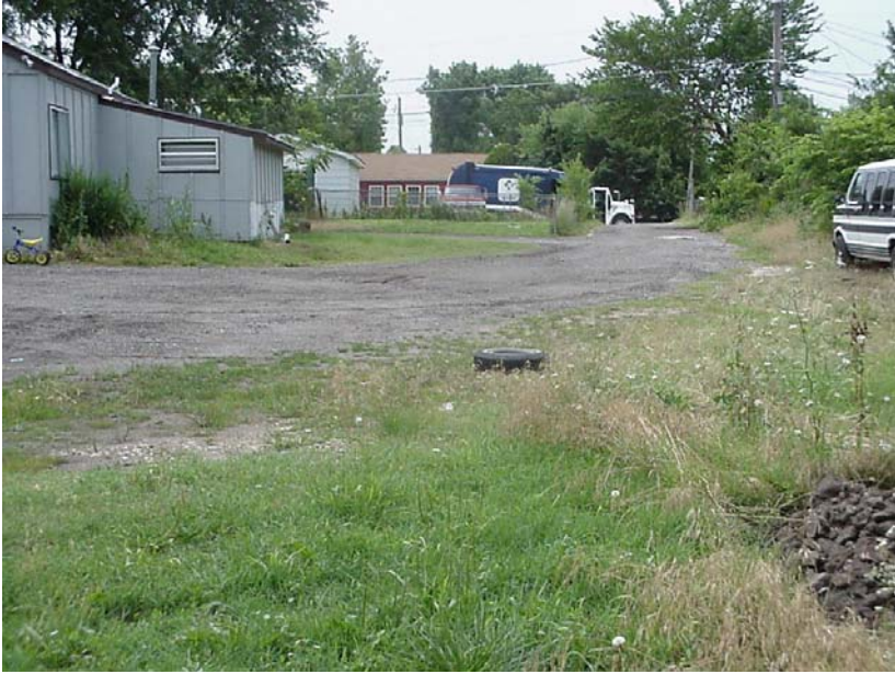
I'm standing on MH 5744-688, looking south. Restoration of gravel/asphalt drives is incidental to pipe replacement.
