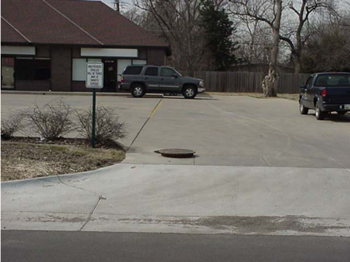
Standing in Joann Street, east of MH 5248-349, looking west. The entire point repair is within the concrete parking lot.
