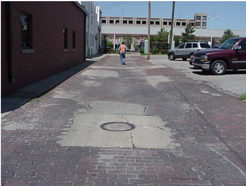
I'm standing south of MH 5547-042, looking north. Shows brick alley & existing patches.
