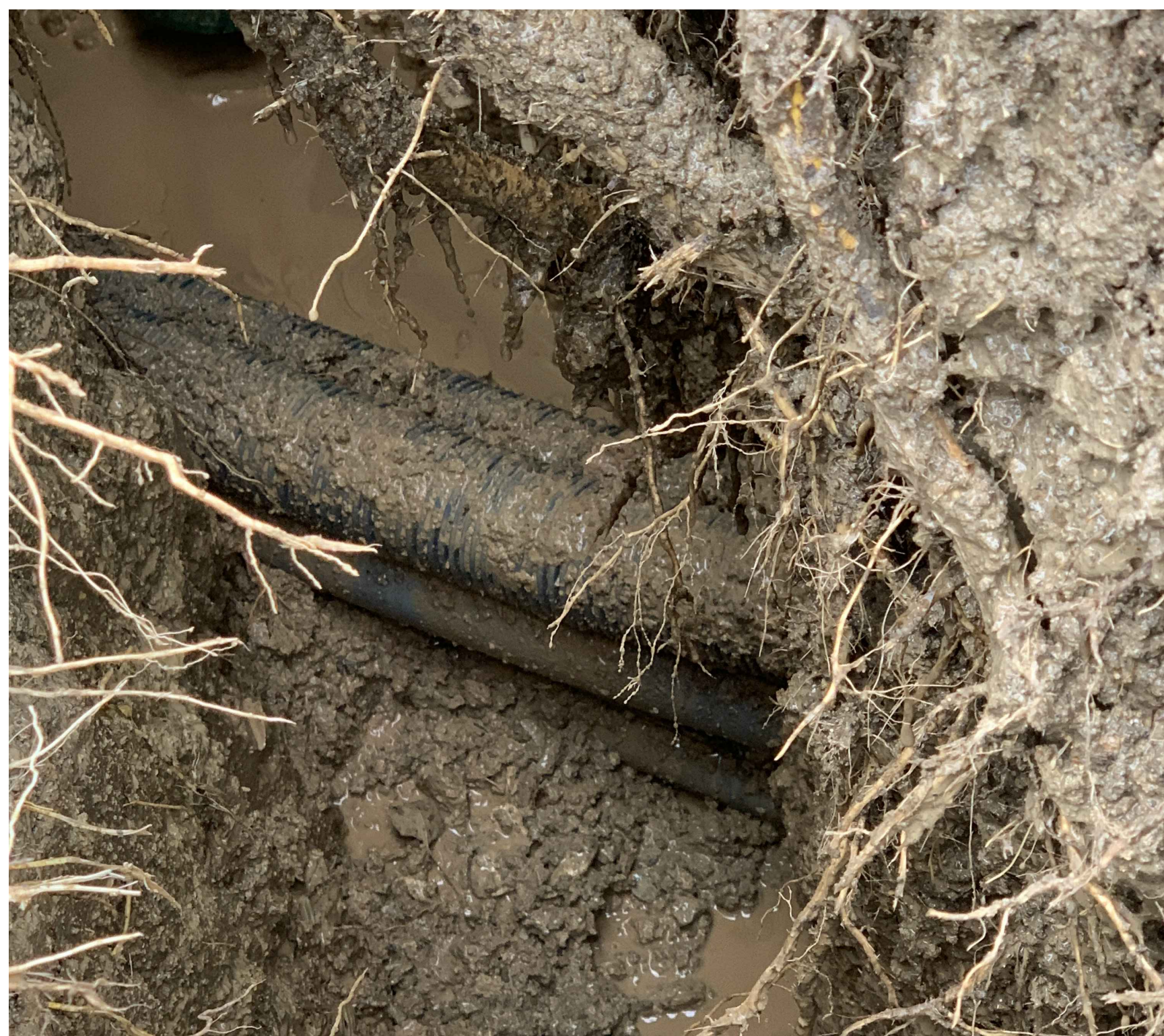
Exposed electric and communications lines near connection point.
