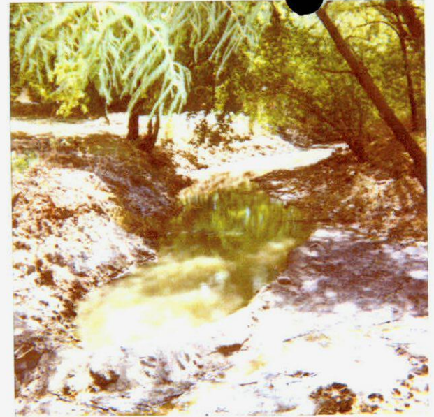
7. VIEW IS RECENT EXCAVATION OF EAST BRANCH OF GYPSUM CREEK AT CONFLUENCE WITH POND OUTLET CHANNEL
