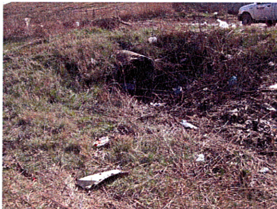
Photo #17 View of roadside ditch and culvert located on the western boundary of the site near underpass of Hydraulic Street and I-135.
