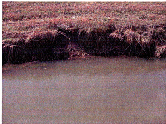
Photo #6 View of typical eroded bank along drainage ditch.
