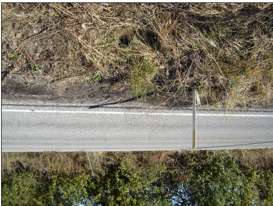
Plugged up 24" CMP under 23rd Street South
