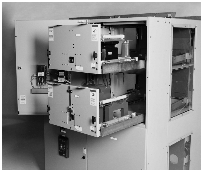
Figure 23. Typical VT and CPT Drawer in the Upper Drawout Position.
