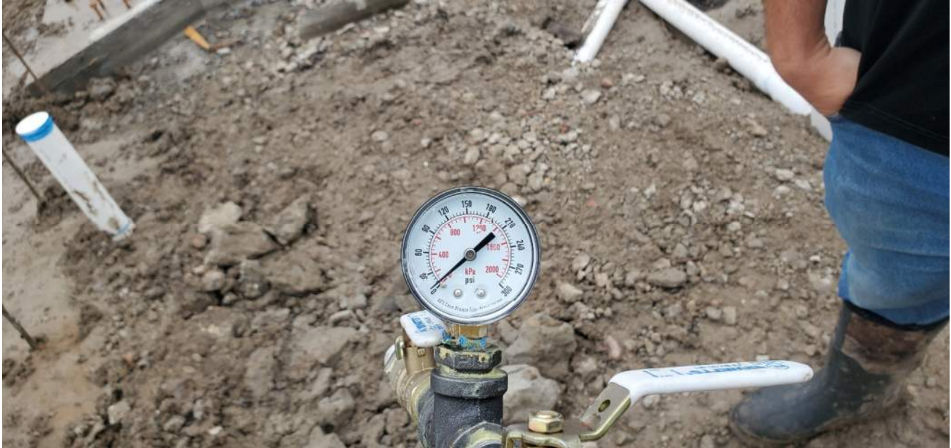
Gauge zeroed at the end of the hydrostatic pressure test.
