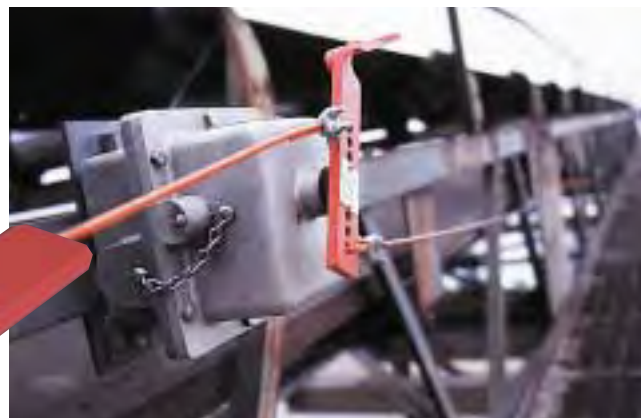
The model RS Safety Stop Switch in operation for immediate shutdown of conveyor system at a sand and gravel company.
