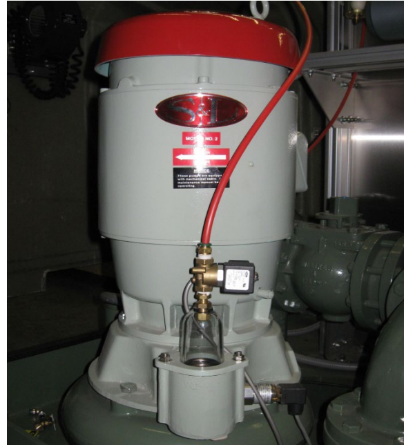
5.14 Main Pump Motor
