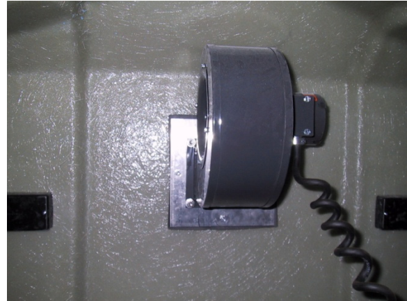
Picture 5.2 Fan Installed In Station Enclosure
