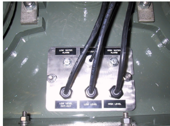
Picture 3.1 Float Switch Cover Plate with Cables Installed on Baseplate.
