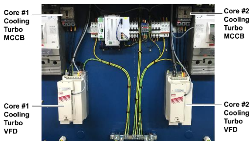
Fig. 17: Frequency converter for cooling air system
