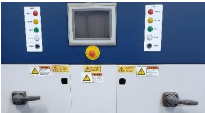
Fig. 91: Main circuit breakers
