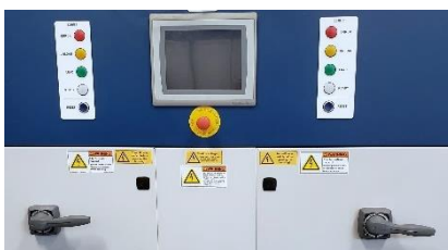
Fig. 63: Main circuit breaker
