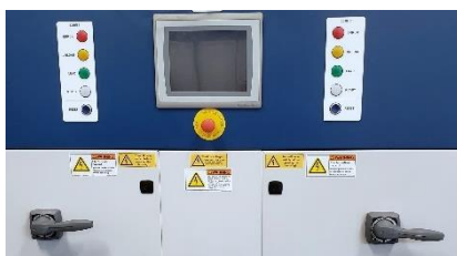
Fig. 90: Main circuit breakers
