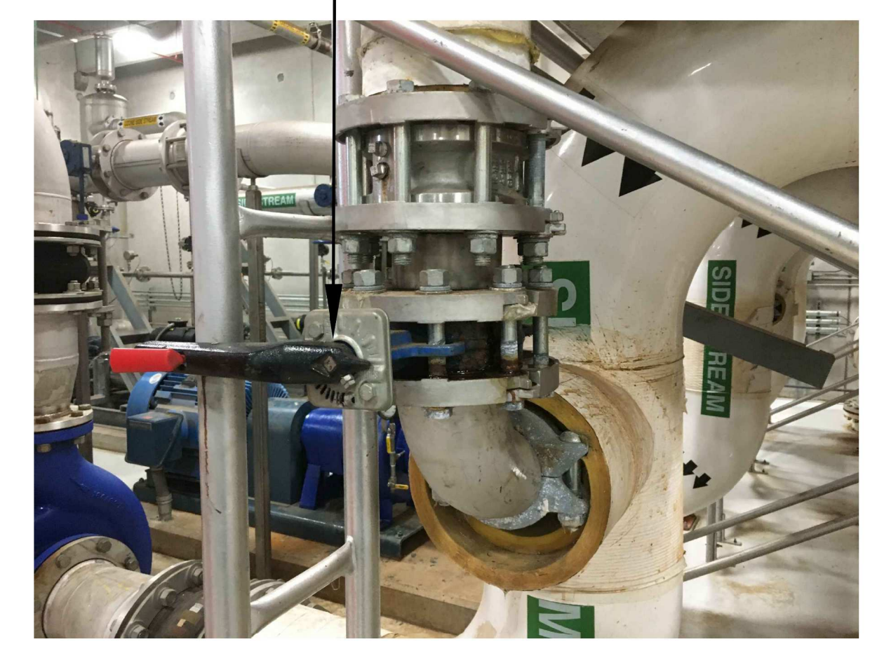
3 4" WATER SUPPLY VALVE C-102
