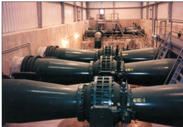
Ball valve in distribution pump station.
