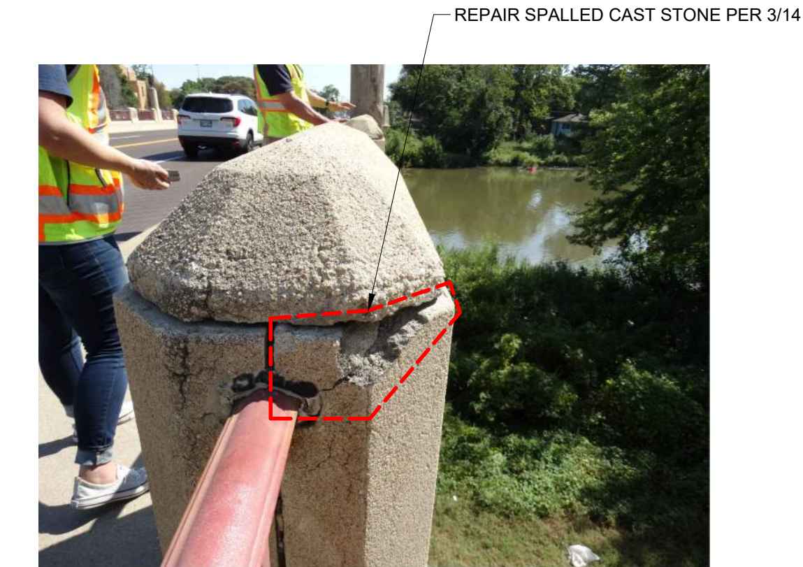
REPAIR SPALLED CAST STONE PER 3/14
