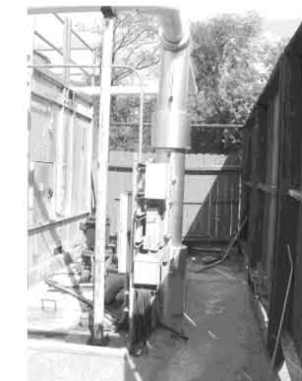
EXISTING COOLING TOWER EQUIPMENT
