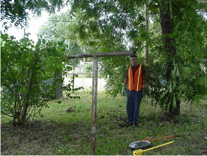
This guy is standing at cleanout/bend (5744-798CO) Measures out to be 17 ft west of the west line of the house and 39 ft north of MH 5744-799
