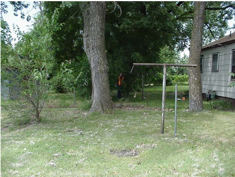
I'm standing south of MH 5744-799 (shown), looking north toward the guy that is standing at cleanout/bend 5744-798CO.
