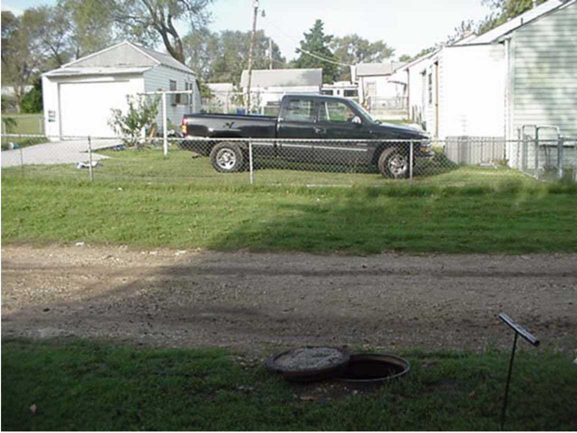
Standing east of MH 5744-684, looking west. Pipe goes between two buildings. Contractor should review the site.
