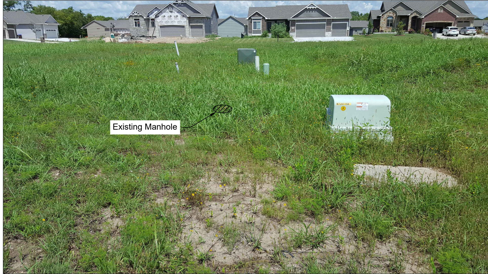
Figure 1 Photograph of MH 1-0 from the south, viewing toward the north. Note the nearby utility structures. See Sheet 6.
