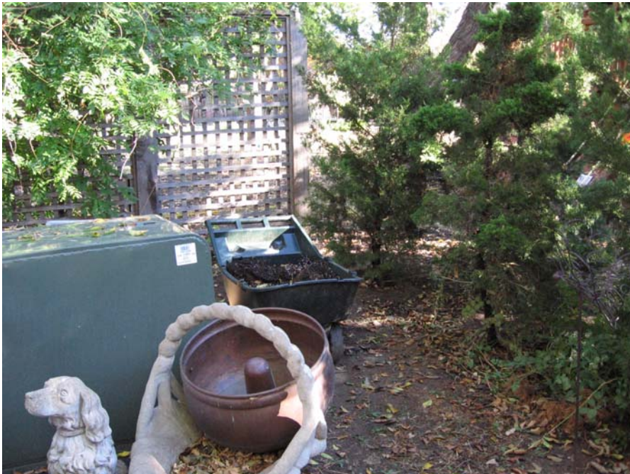
Standing south/southwest of the excavation site, looking northerly. There is a transformer box in the vicinity, so the manhole will be constructed fairly close to the south side of the lattice fence (northeast of the transformer box).
