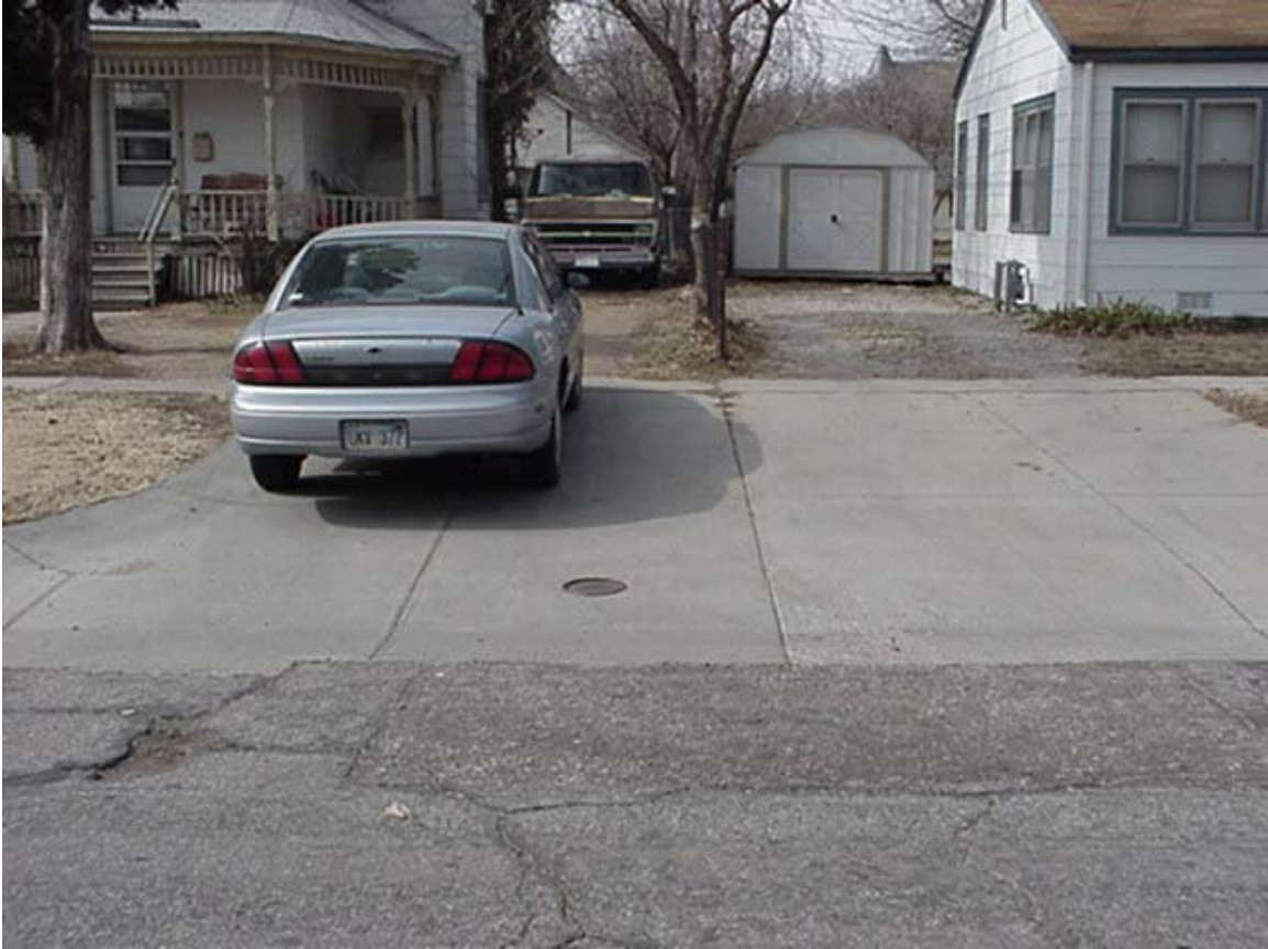
Standing in Glenn Street, looking west. New MH 5346-135 should have the lid centered in the sidewalk.
