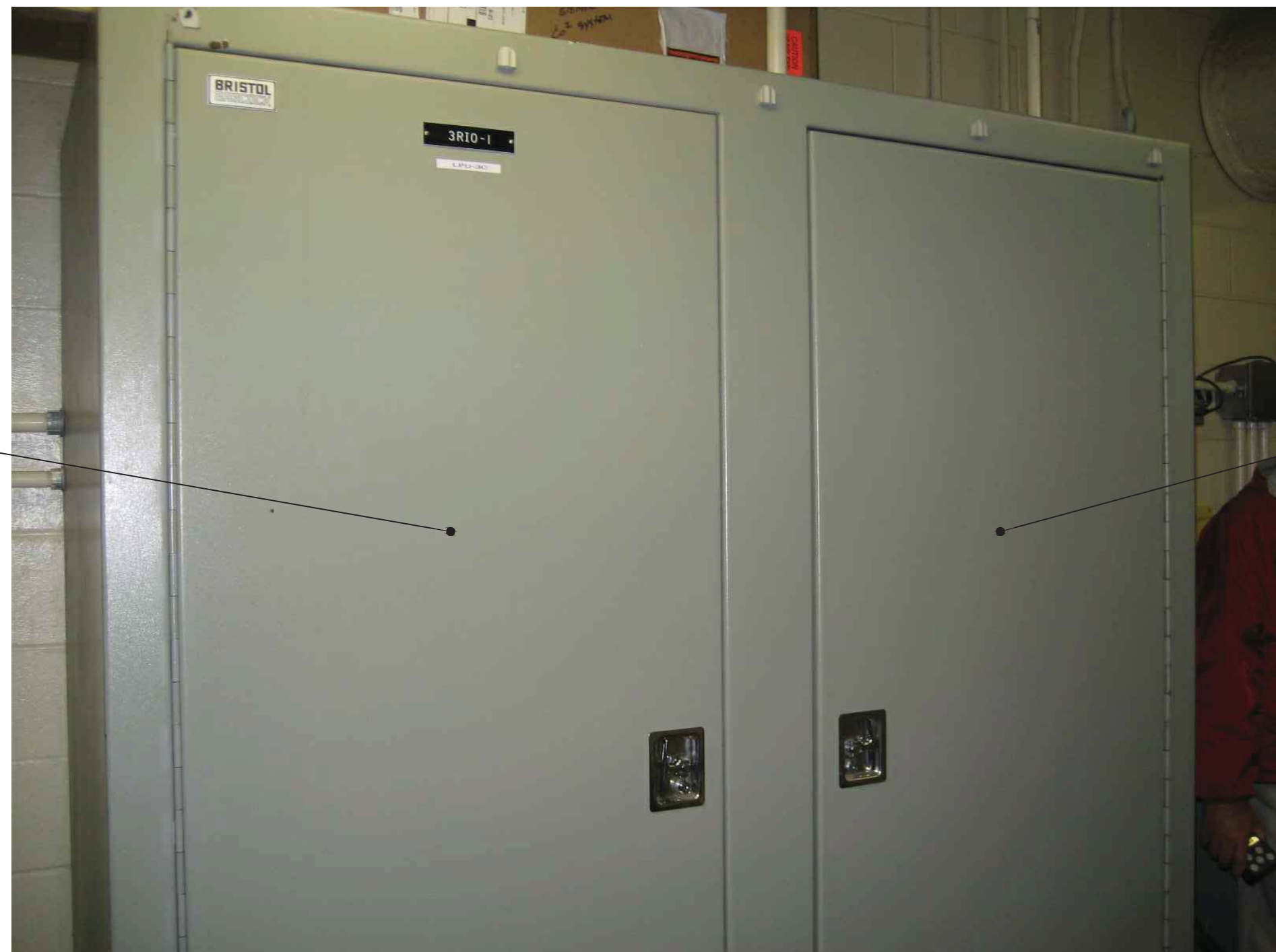
PHOTO 1 - 3RIO-I PLC CONTROL CABINET NOT TO SCALE
