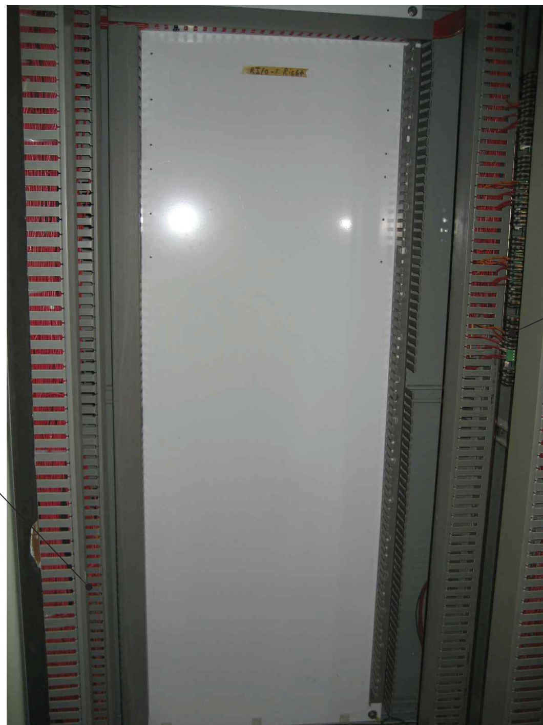
PHOTO 2 - PLC CONTROL CABINET INTERIOR NOT TO SCALE
