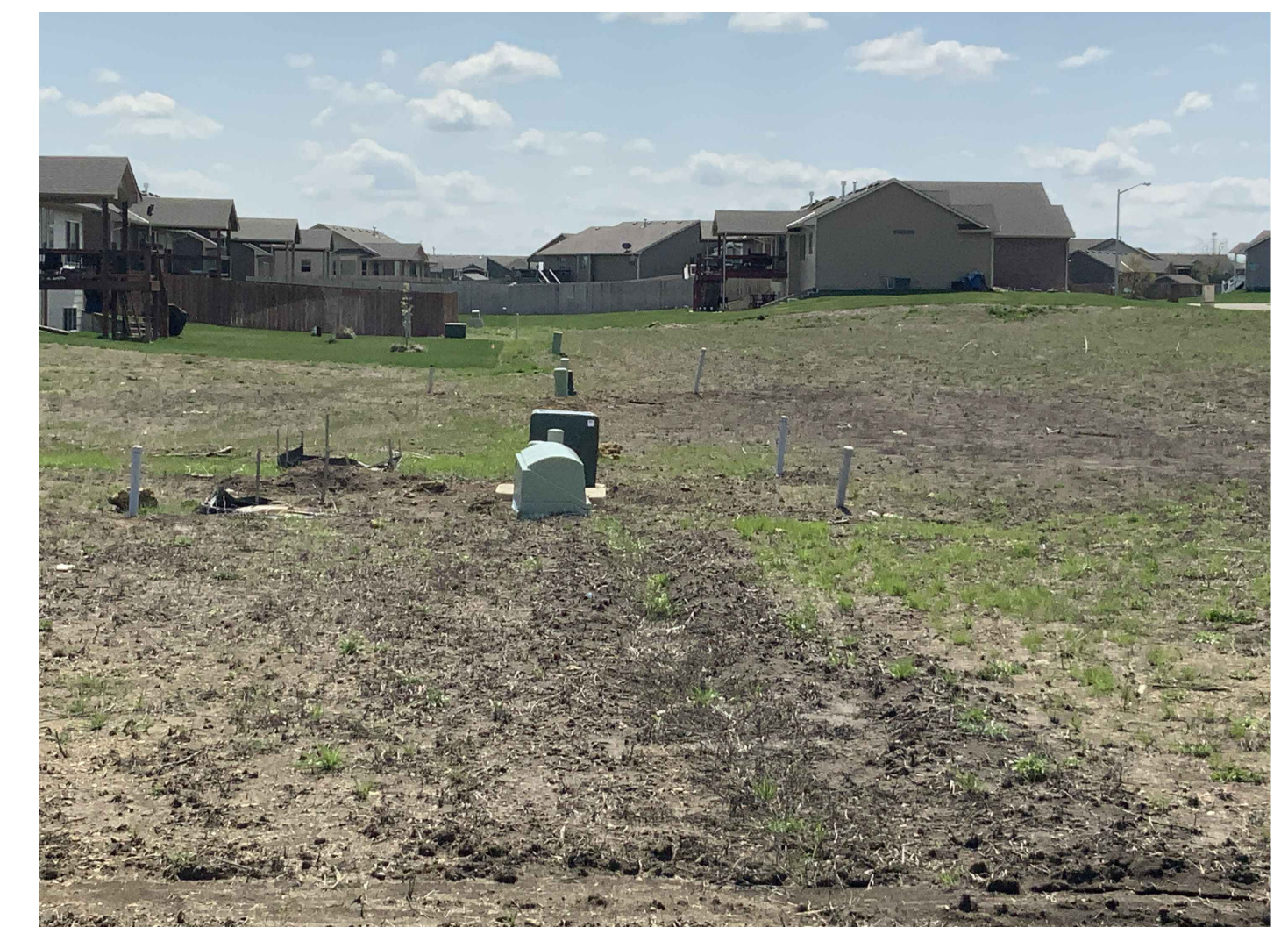
*P: The backyard easement of Block 4. Note that all utilities are installed. Use caution when grading. Do not damage structures in this or any other easement.
