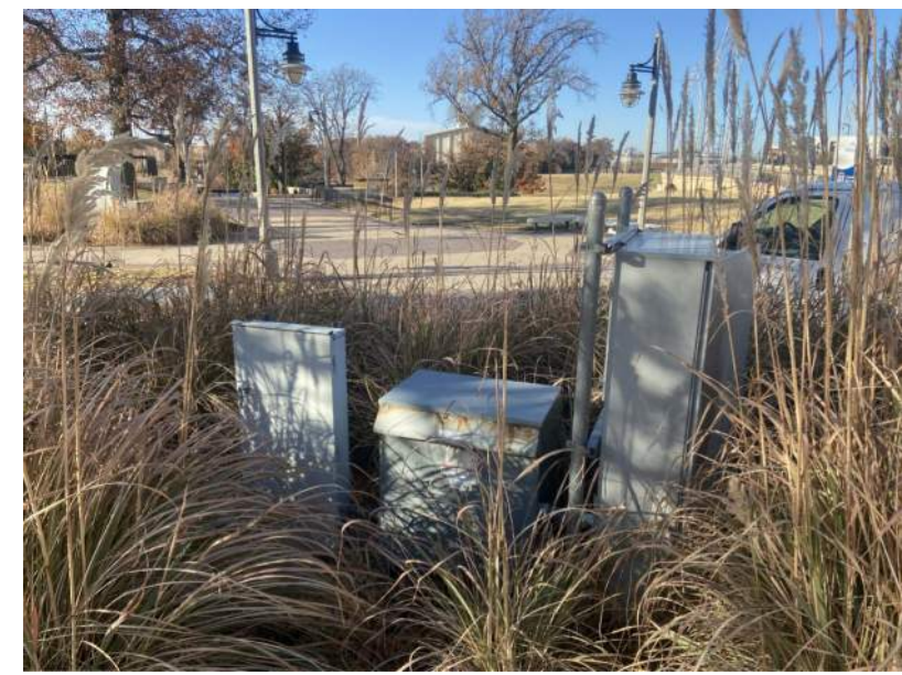
EXISTING PANEL 480' and 208'
